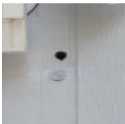
Carpenter bee damage
