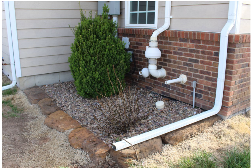
Figure 3. Pea gravel placed in a planting area to reduce clover mites from entering (Raymond Cloyd).
